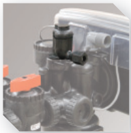
The chlorine generator valve disinfects when iron or sulfur bacteria might be present.
