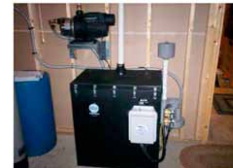
Radon Mitigation System
